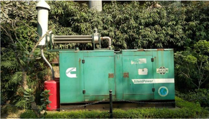
A Chakr Shield attached to a diesel generator
